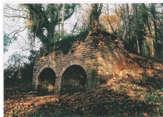
Damage to lime kiln due to vegetation growth – root system forcing out stonework – long standing issue but damage is active and ongoing
