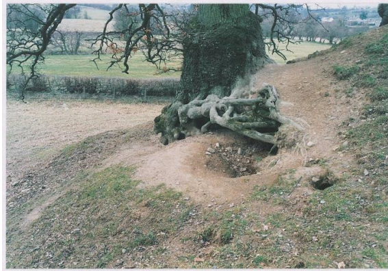
Multiple issues – tree root damage (long standing) plus badger damage & stock wear
